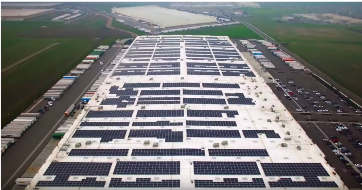
Amazon Warehouse Rooftop Solar Panels (Photo from cnet.com )
