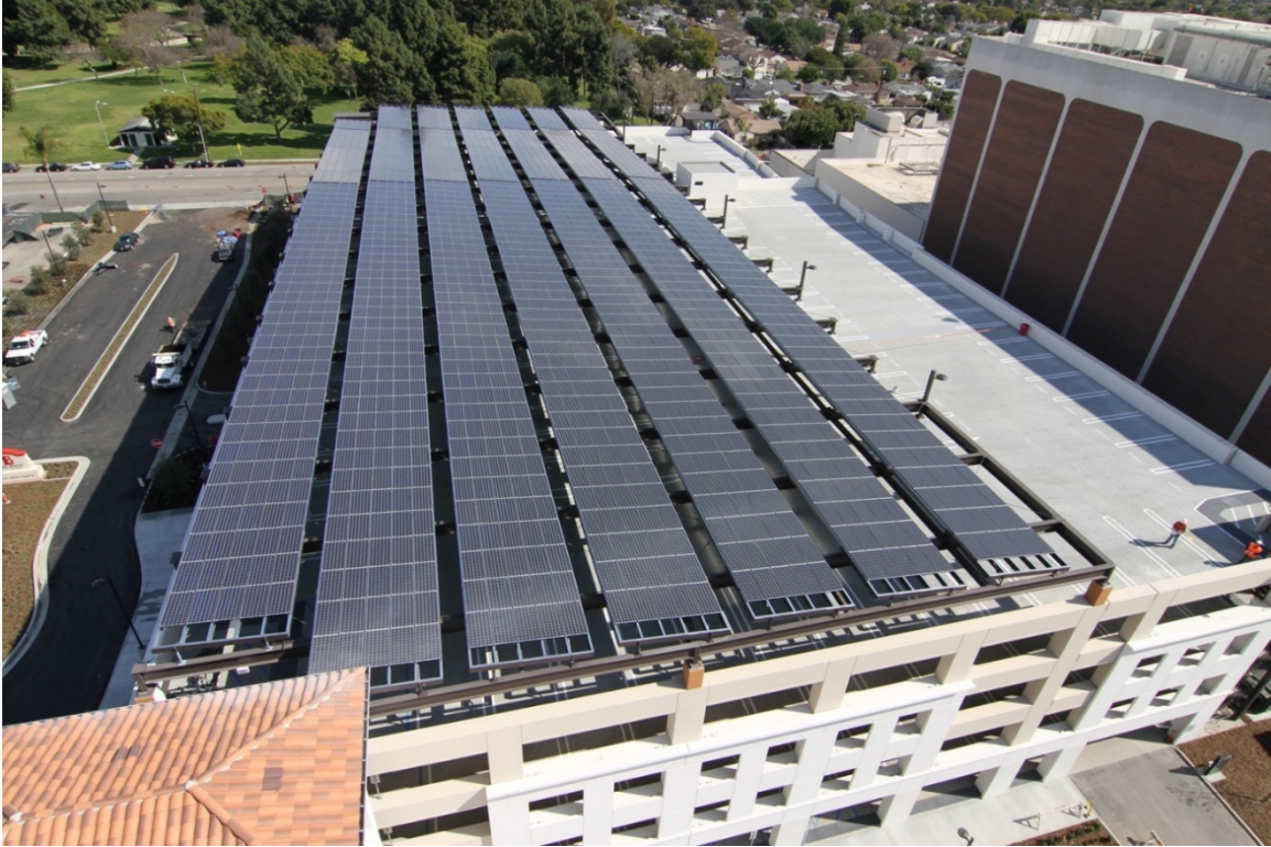
Parking Deck coverage that still allows vehicle parking underneath the solar panels at Long Beach City College (Photo from greenbuildingelements.com )
