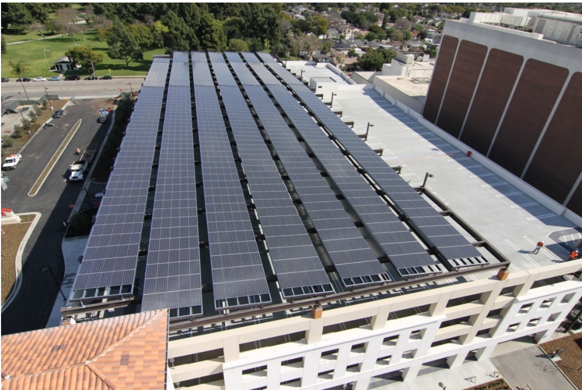
Parking Deck coverage that still allows vehicle parking underneath the solar panels at Long Beach City College (Photo from greenbuildingelements.com )
